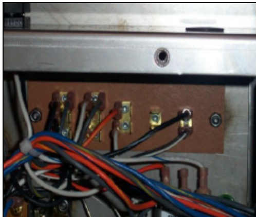
Terminal board inside the heater box
