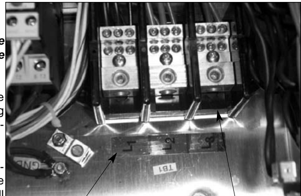
Incoming Power Connection
