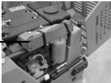
Figure 10. Location of Remote Control Cable
