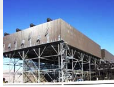
Big Horn Nevada, USA — ACC for 500 MW Combined Cycle Power Plant
