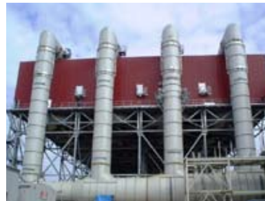
Astoria New York, USA — ACC for 500MW Combined Cycle Power Plant
