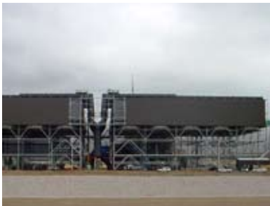
Silver Hawk Nevada, USA — ACC for 500 MW Combined Cycle Power Plant
