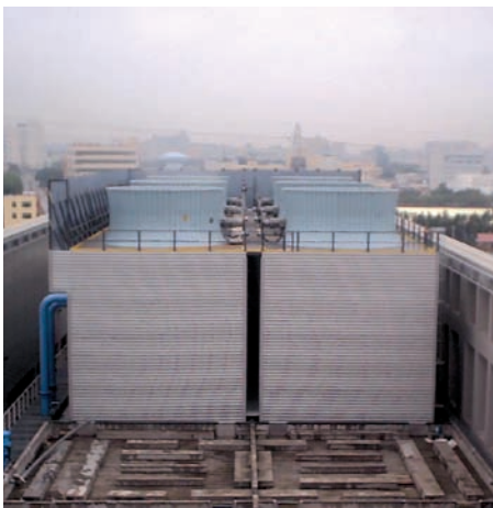
➤ Class 400 cooling towers in Taiwan
