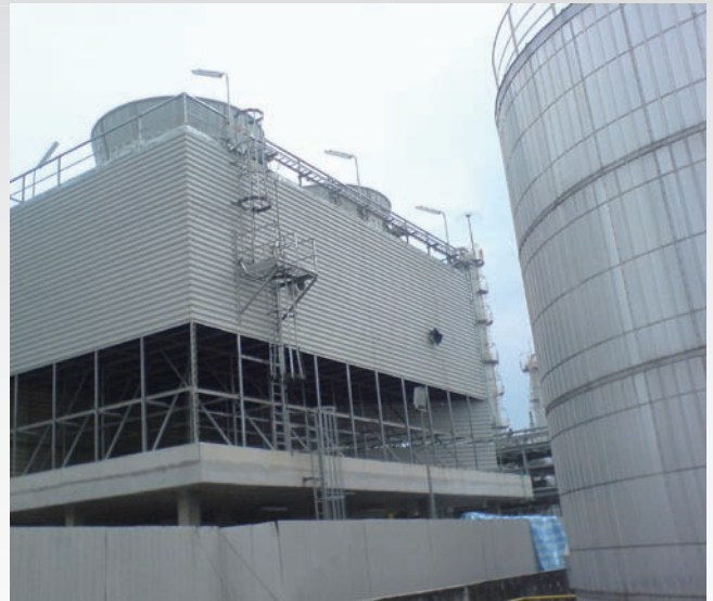
➤ Class 400 cooling towers in Singapore
