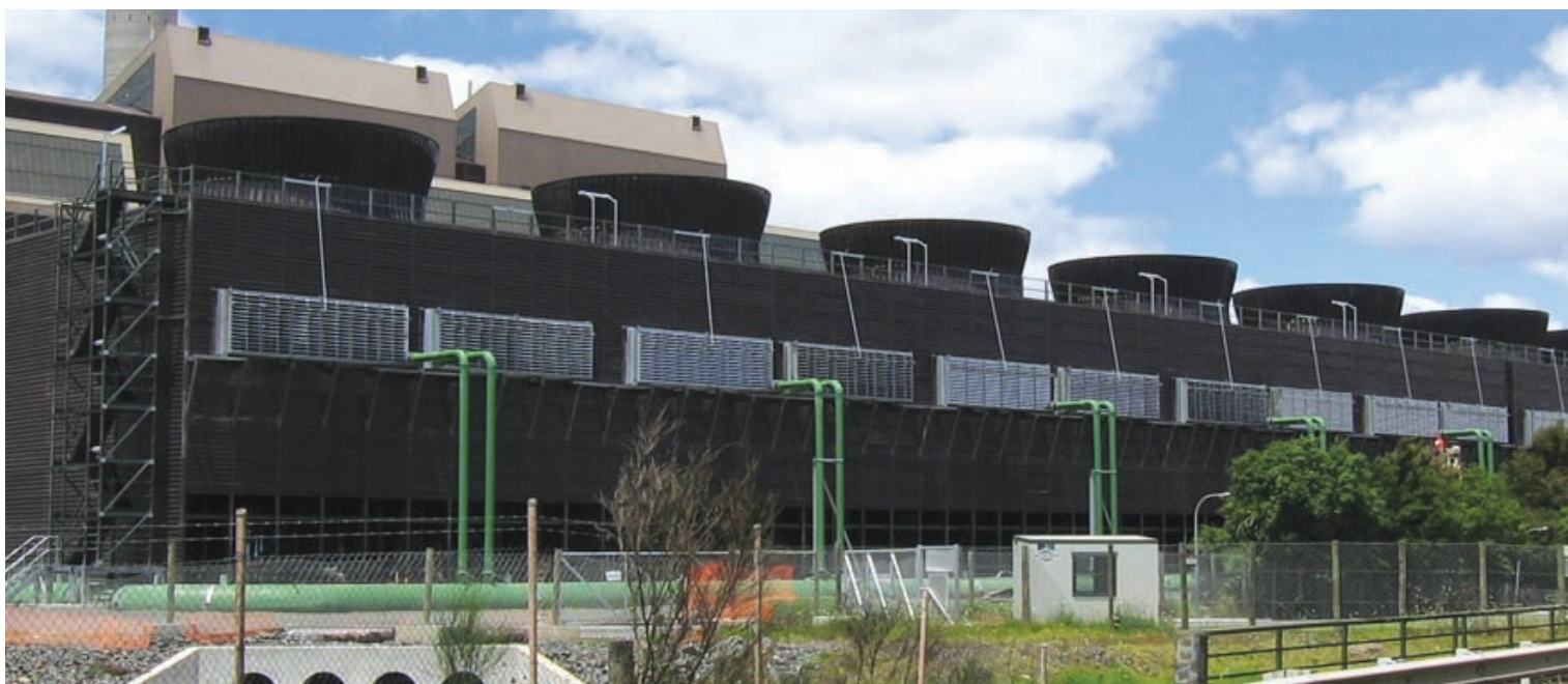
Class 400 cooling towers in New Zealand
