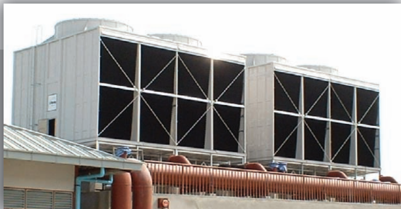
► NC Fiberglass cooling towers in Thailand
