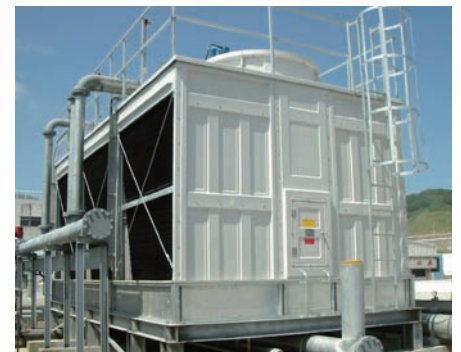
▶ NC Fiberglass cooling towers in Hong Kong
