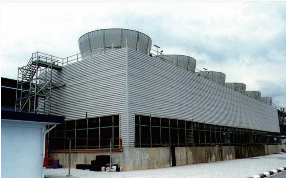
▶ Class 400 cooling towers at KLIA in Malaysia
