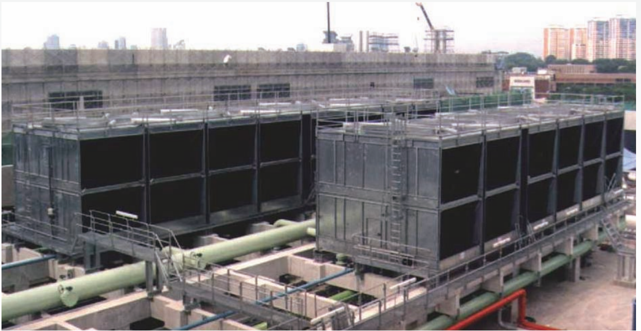
➤ NC Class cooling towers in Singapore
