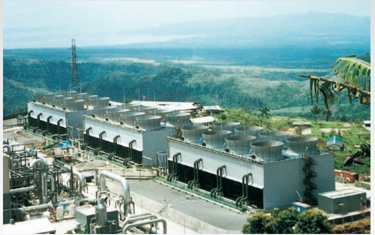
Class 400 cooling towers at Geothermal plant in Philippines
