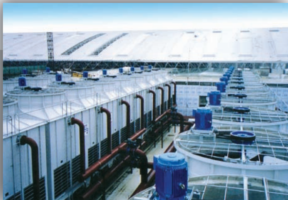
➤ SRC cooling towers in China
