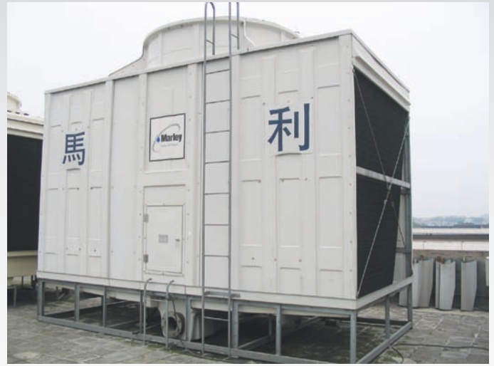
➤ NC Fiberglass cooling tower
