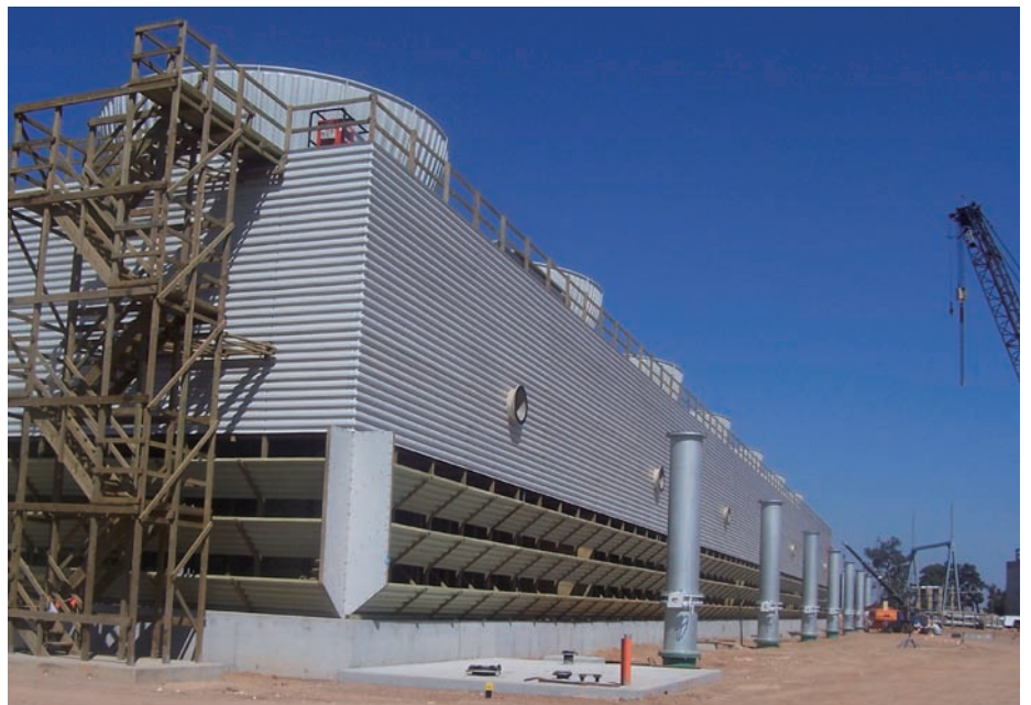
➤ Class 400 cooling towers in Australia
