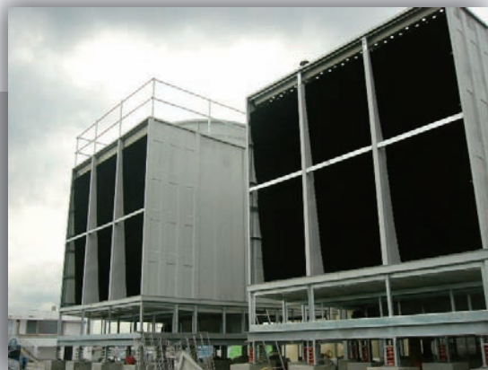
➤ NC Fiberglass cooling towers in Singapore
