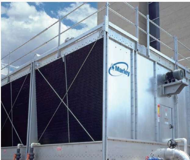
➤ NC Class cooling tower
