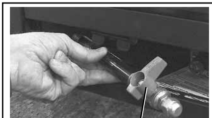
Length of pipe with attached Gas Shut-Off Valve in OFF position (gas line CLOSED)
