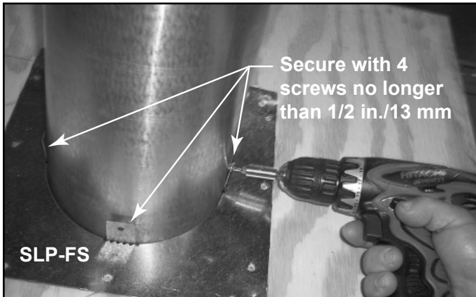
Figure 10.18 Secure Pipe with SLP-FS
